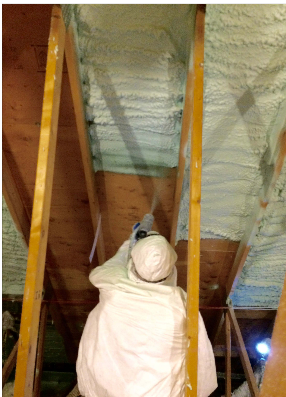
The Town of Macedon offices will be closed Thursday (10/29) and Friday (10/30) as work proceeds on the $900,000 Trane project that the Town coupled onto with the County. The energy saving project will spray-insulate the building, install new LED lighting and furnaces. The Trane Company guarantees energy savings that will save the Town the cost of the work over a 16 year commitment. The Town Library, next door to the Town Hall, had the insulation blown in this past week.
